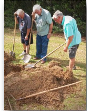
Jim Johnson, Charles Pennington and Ron Allen "look" for Tom Carter while repairing another water leak. (Photo by Chris Allen)
