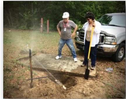
Tony and Pam enjoy finding the major water leak geyser. Several volunteers dug for part of three days trying to locate it. Thank you ALL!
